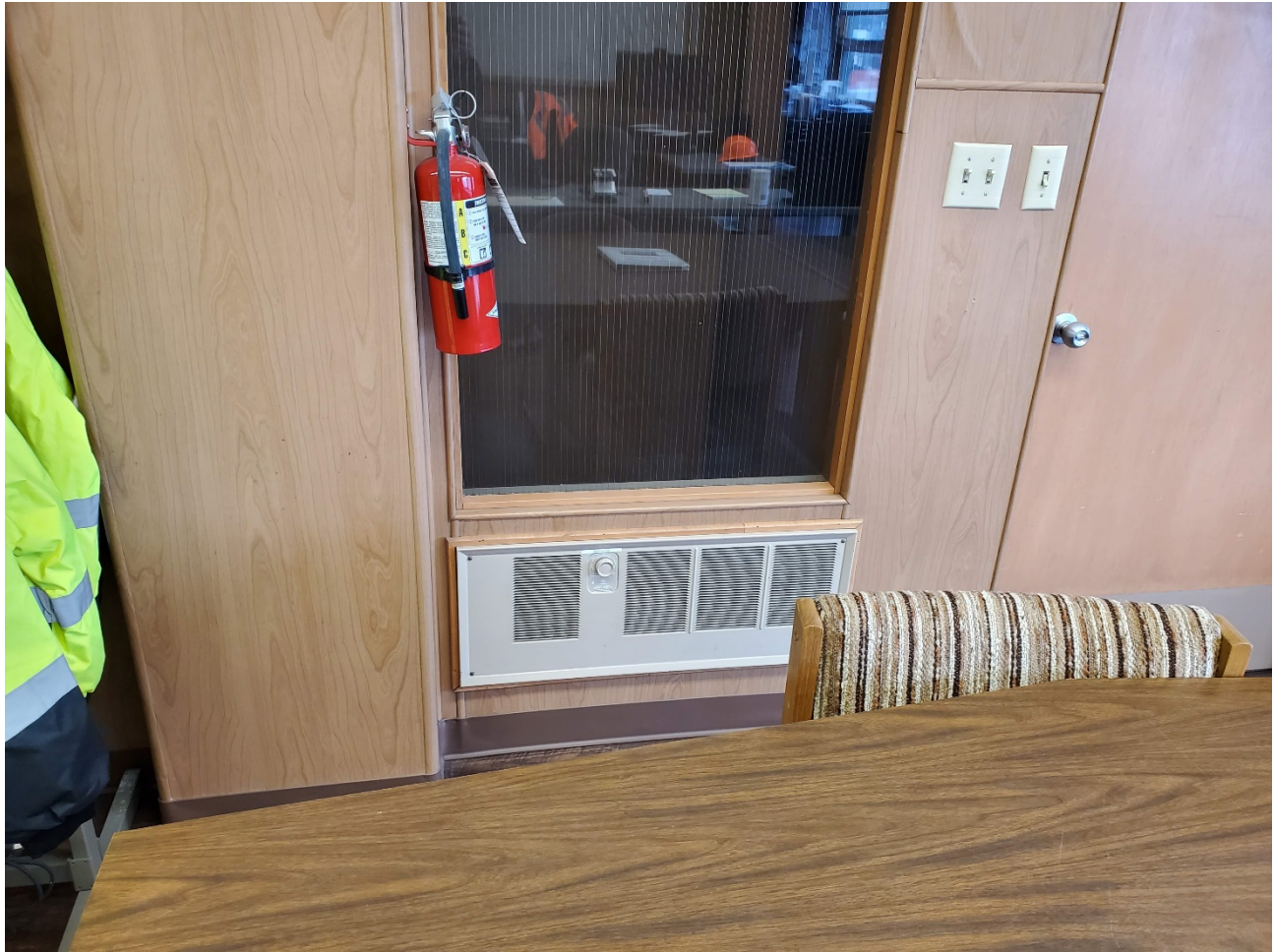
Figure 3- Marine Terminal Back Office Cadet-Style Heaters
